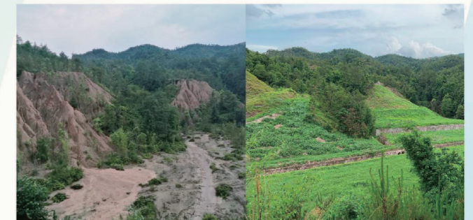
赣县区大田乡废弃矿区重金属综合治理工程（一期） Phase I Project for Comprehensive Treatment of Heavy Metals of Abandoned Mining Area in Datian Township of Ganxian District
