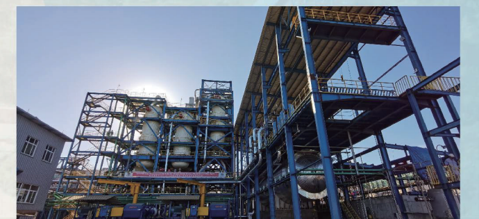
印尼OBI红土镍矿湿法冶炼项目 Project of Nickel Laterite Hydrometallurgy of OBI in Indonesia
