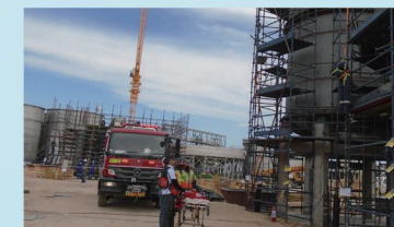
项目现场举行应急演练 Emergency drilling held on the project site
